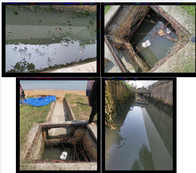
Figure 2 Cloudy green water from drainage to outfall at the Port Dickson beaches.
